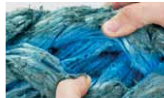
Inspect for internal abrasion.
