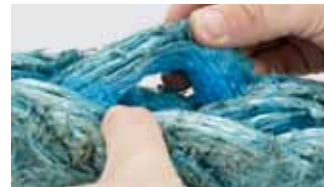
Inspect for pulled strands.
